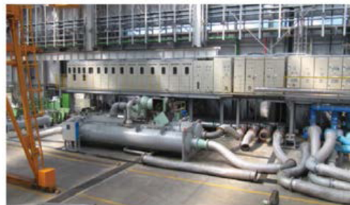
Performance test facilities
